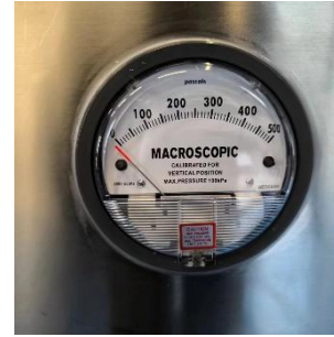
Differential pressure gauge
