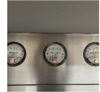
Differential pressure gauge
