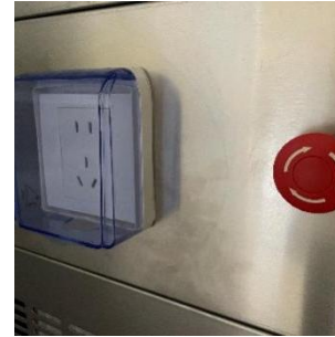
Sockets and emergency stop
